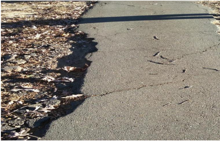
Cart path on #14 that needs repair.
