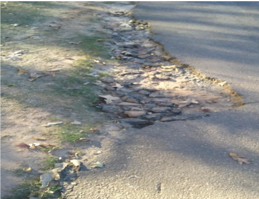
Cart path on #11 that needs repair.
